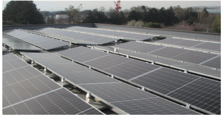
Solar panels at the Saitama Factory
