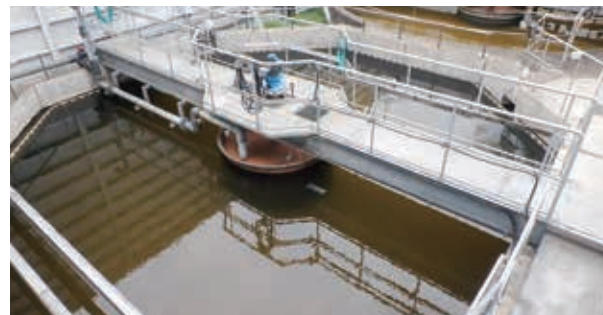
Wastewater treatment equipment at the Saitama Factory
